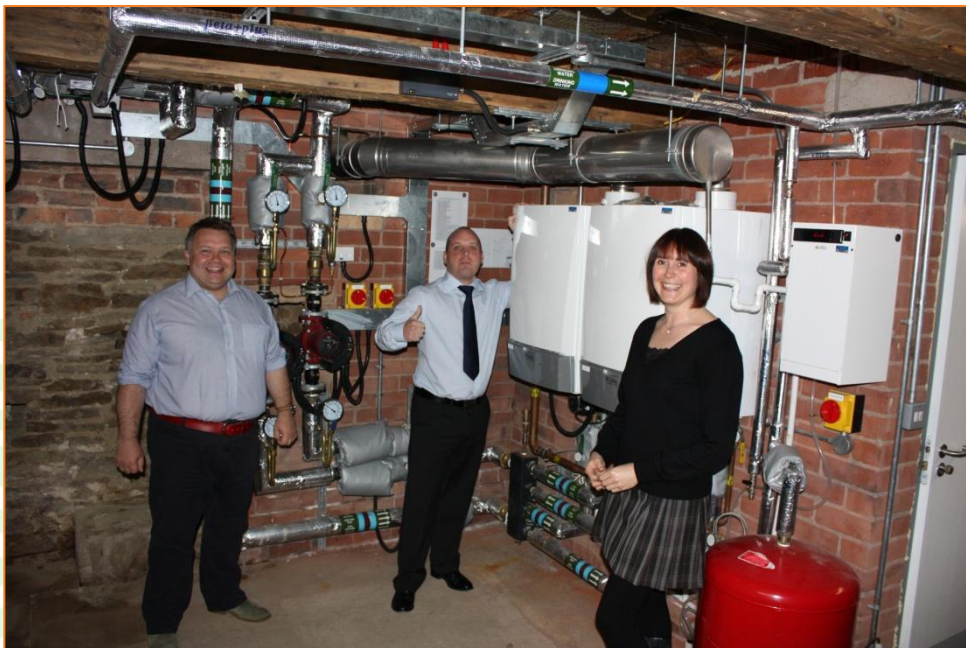
Feeling hot, hot, hot (well, hopefully not!): Ian Palmer, John Walker and Ruth Lilley show how excited the team at Barber House are about their new boiler
